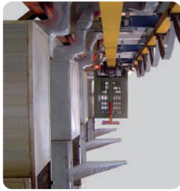
Central Portering System and Central Furnace
